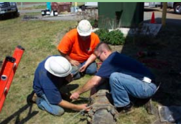
Well 8 Water Main Break
