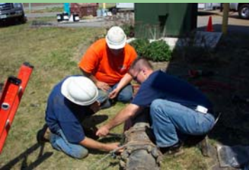
Well 8 Water Main Break
